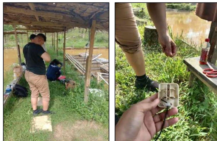
Figure 5. Aerator Team and Electricity Team at work (left side) Figure 6. Terminal Electricity Manufacturing for Oxygen Pump (right side)
