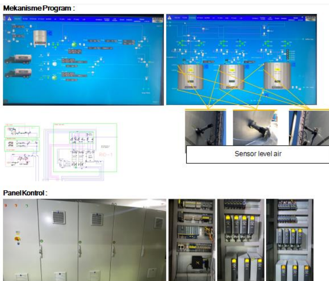
Gambar 1. Integrated Automation Pump
