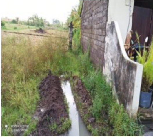
Figure 2 Irrigation channel damaged due to housing development
